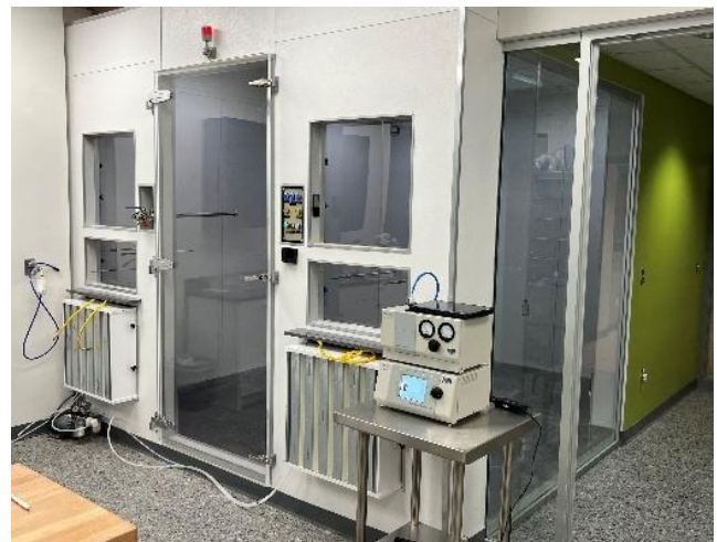
Figure 3: The 30 m 3 bioaerosol testing chamber at ARE Labs adheres to AHAM AC-5 standards and ASHRAE 241 criteria. The chamber is equipped with HEPA filtered air in/out, multiple bio aerosol sampling ports, decontamination, and pressure balance.
